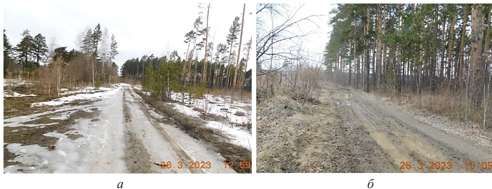
Рис. 4. Состояние поверхности дороги на 26.03 на участках: a – № 3; б – № 4 Fig. 4. The road surface condition as of March 26 in sections: a – no. 3; б – no. 4
